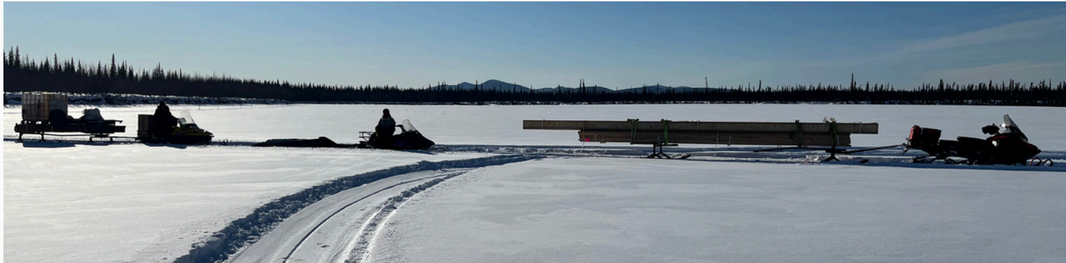
Hauling out the 32' I joists and other supplies for the Lodge addition
